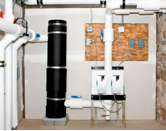
A geothermal system at The Lodges at Gettysburg heats and cools a lodge building.
